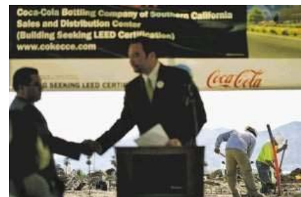
Construction work continues in the background as Coachella Mayor Eduardo Garcia (left) shakes hands with Coca-Cola San Diego market unit Vice President Ken Ramirez during a groundbreaking ceremony on Feb. 19 for the environmentally friendly Coca-Cola Bottling Company of Southern California Sales and Distribution Center in Coachella. (Crystal Chatham, Desert Sun file photo)
