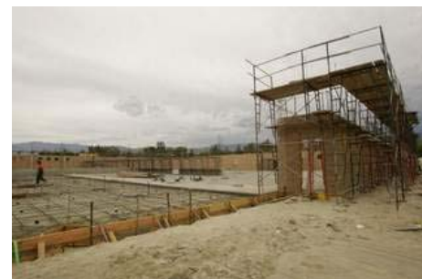
Construction was under way June 3 on the Riverside County Sheriff's Department's new 85,000-square-foot Palm Desert station along Gerald Ford Drive in Palm Desert. The building is designed to meet LEED gold certification. The building will have photovoltaic solar panels, energy-efficient windows and air conditioning, skylights, and water-efficient drains and toilets. (Crystal Chatham, The Desert Sun)
